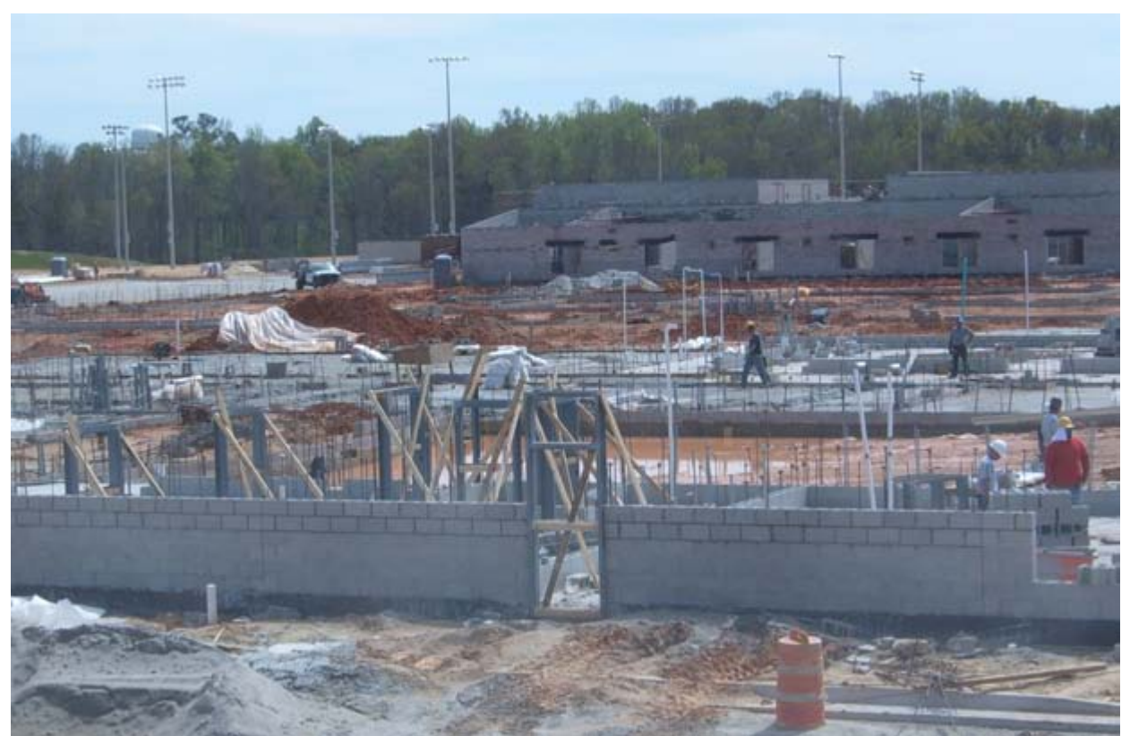
Work is progressing on the new high school, located off of Metasville Road. In fact, the Lincoln County Board of Education voted to sell $15,625,000 in general obligation bonds to help pay for the facility at a meeting held Thursday, March 26. Classrooms are pictured in the foreground, with the gymnasium appearing in the background.
